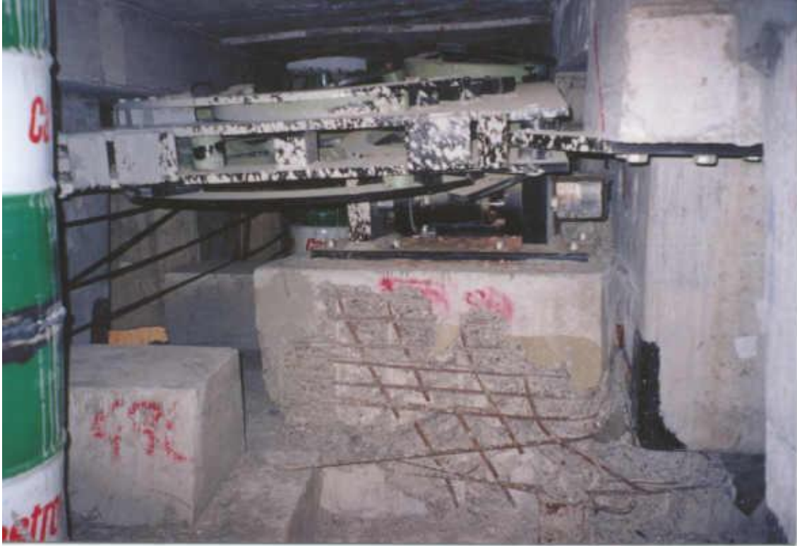
Fig. 5, – Failure of an EDU, damage to EDU support block and Central beam end, due to impact
