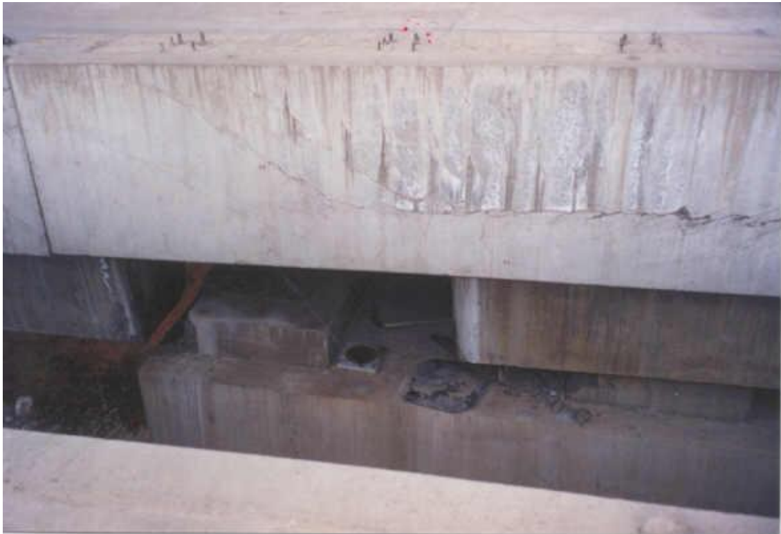
Fig. 6, – Unseating of Beam end at Pier cap
