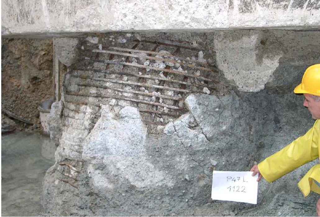
Fig.9, – Extreme example of damage to piles of a foundation on the fault line.
